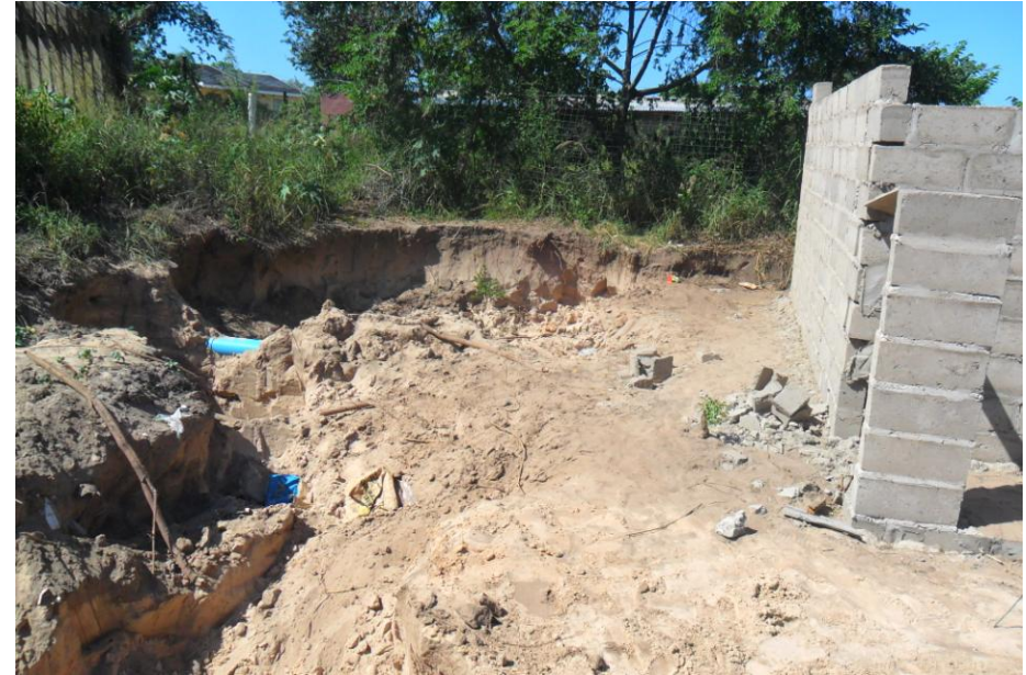
Stopped unauthorised building being erected on top of a sewer pipe from Manguzi Hospital
